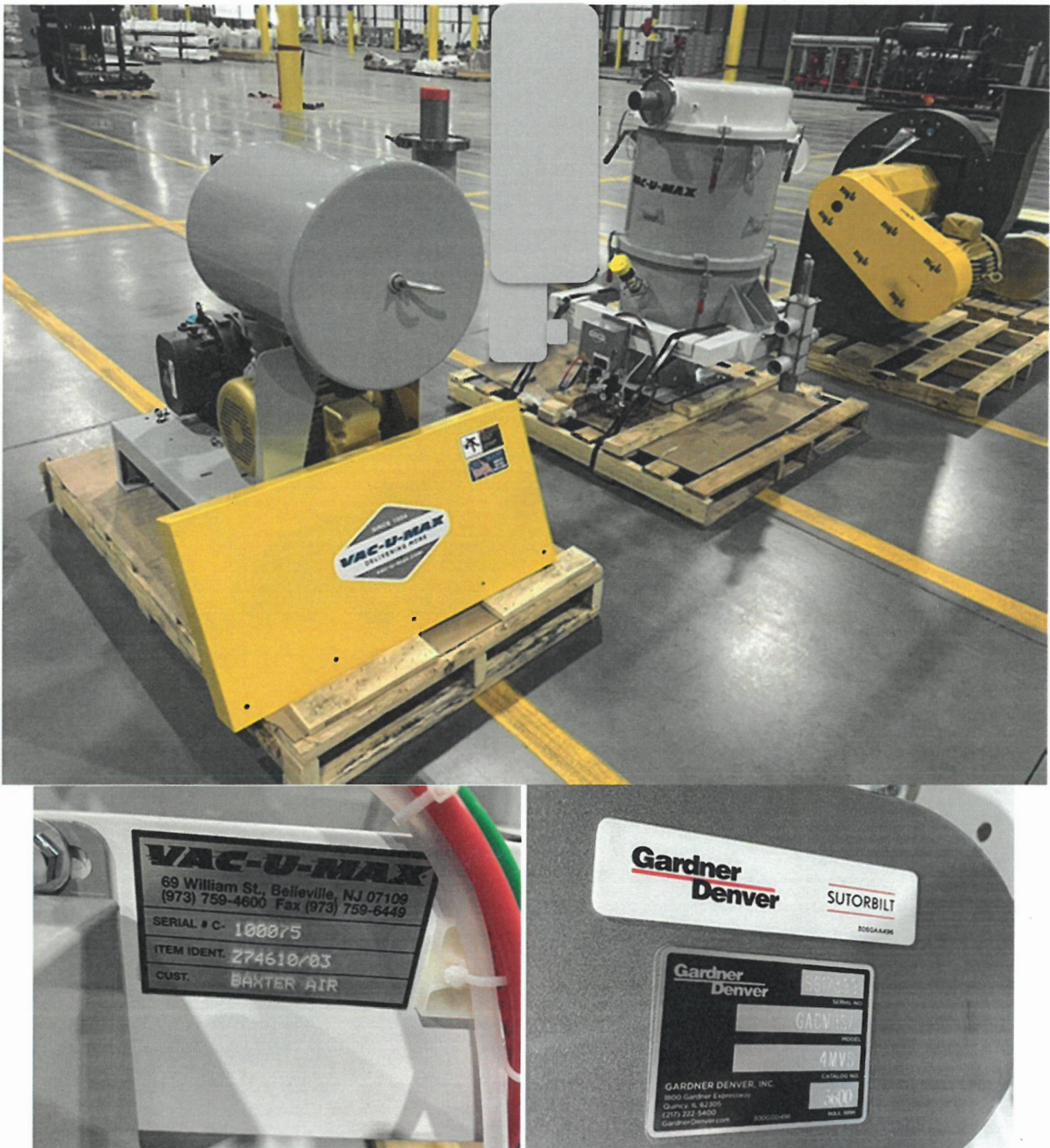
Figure 8: Filter receiver VAC-U-MAX for spent pellet cyclone (Unit #30) and spent pellet blower (Unit #31) relocated from Extract Plant 2 to Extract Plant 3.
